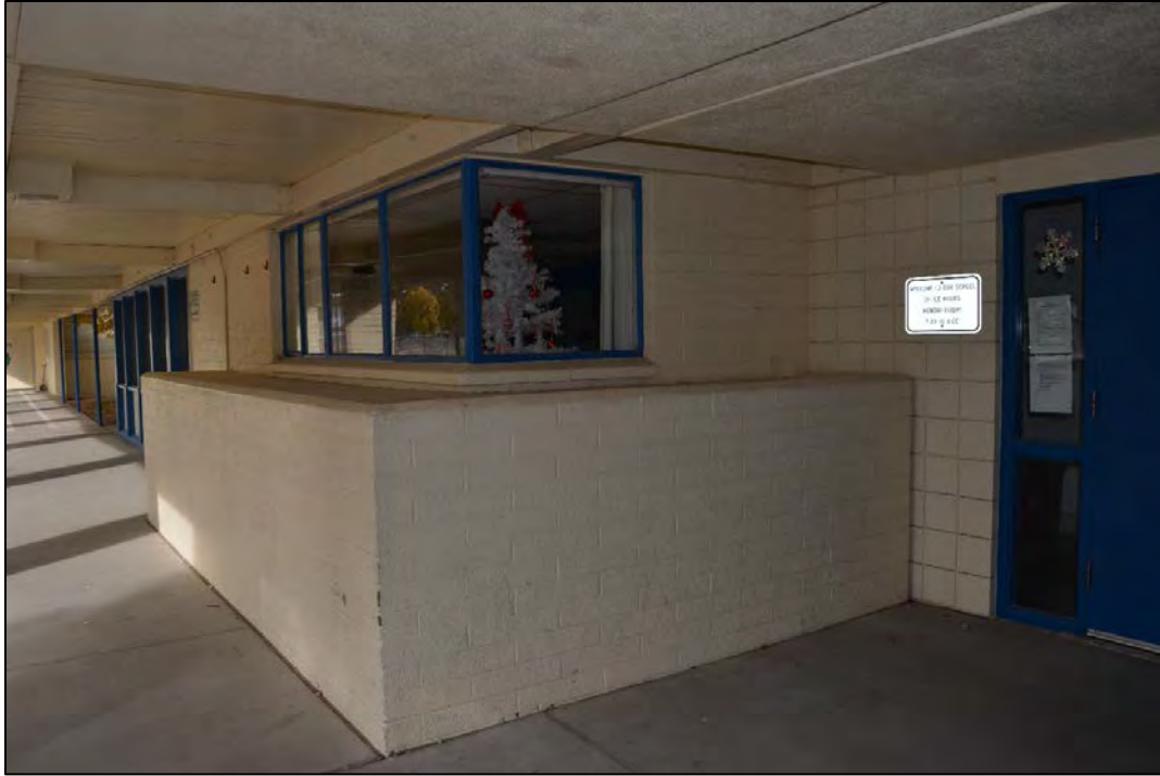
Figure 39. Facility 1781 south elevation, looking northwest. Note: Transition in concrete block dimensions showing the distinction between the original structure and addition. The exterior corner of the 1953 building was converted into a niche within the 1967 addition.
