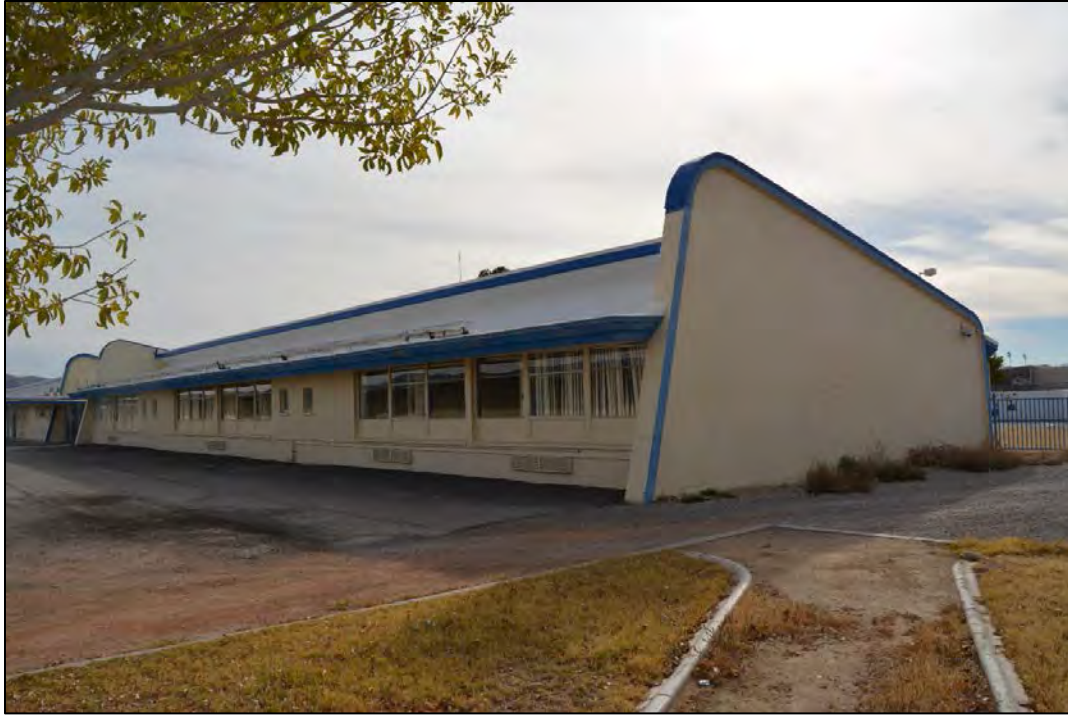
Figure 82. Facility 1789 west and north elevations, looking southeast. Note: Roof windows on the south elevation are covered.
