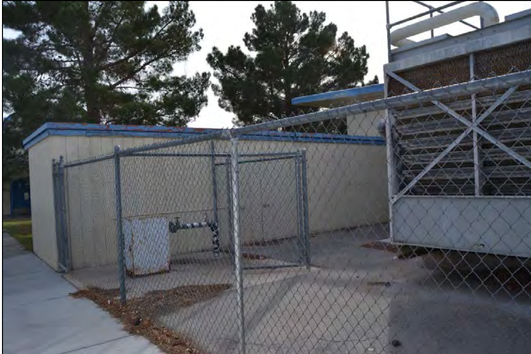
Figure 93. Facility 1790 looking east, the mechanical system is seen on the foreground.
