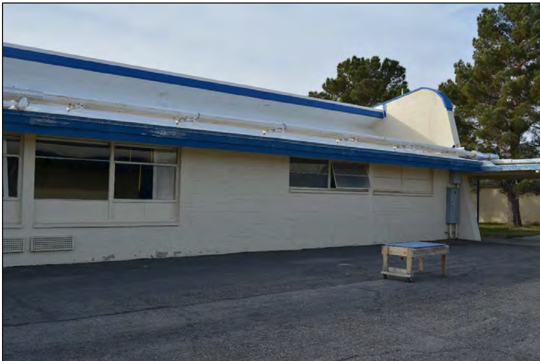
Figure 55. Facility 1783 detail of south elevation, looking southwest. Note: Roof windows are covered (white area under the blue band)
