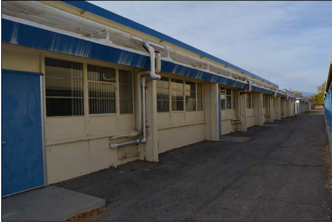
Figure 65. Facility 1785 north elevation, looking southwest. Note: Holes cut in panels beneath the ribbon windows for HVAC pipes.
