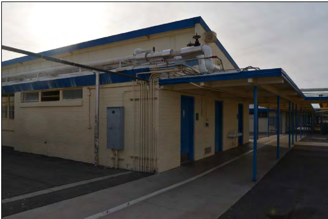
Figure 64. Facility 1785 west and north elevations, looking northeast. Note: Mechanical, electrical, plumbing, and fire suppression systems added along the roofline.
