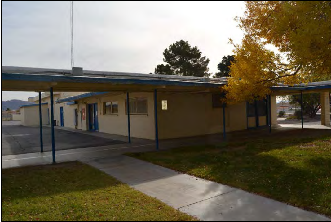
Figure 43. Facility 1781 west and north elevations, looking southeast. Note: Original ribbon windows are located on the north elevation (1953 construction).
